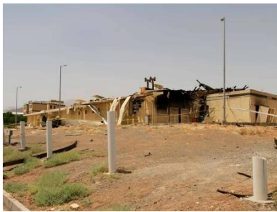
Aftermath of recent explosion at the Natanz uranium enrichment facility (AP)
