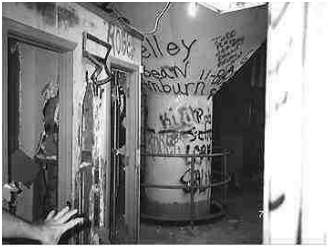
Control Center before Renovation
